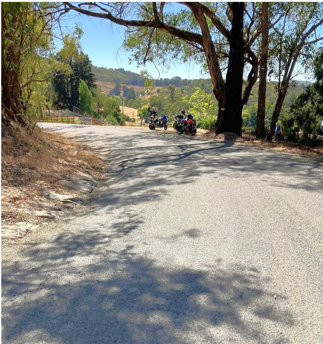
The offending section of road topped with loose gravel
